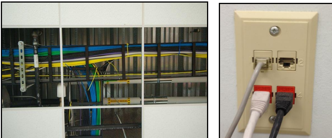
Figure 1: (Left) A typical premise installation with Ethernet cable behind a dropped ceiling and a work area outlet in an office setting (Right)
