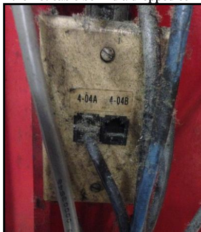
Figure 2: A workstation outlet on a plant floor
